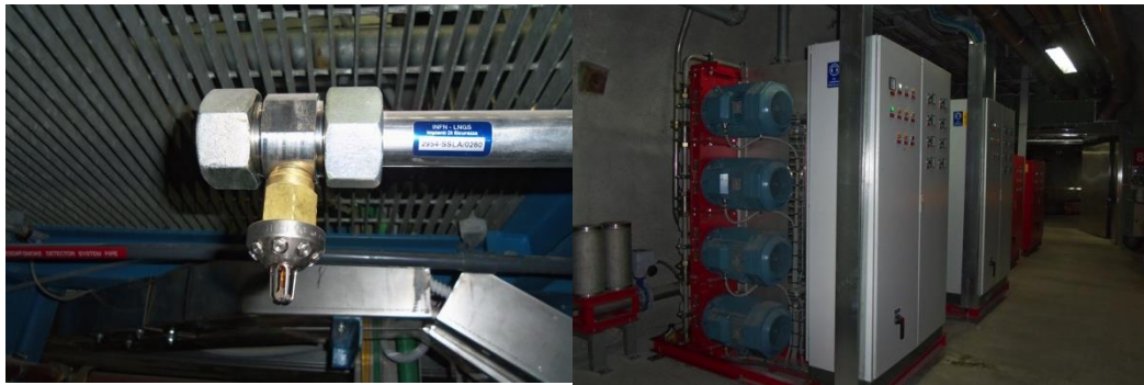
Figure 5.7.2 - Detail of water mist nozzle and pumping units @ INFN-LNGS.
