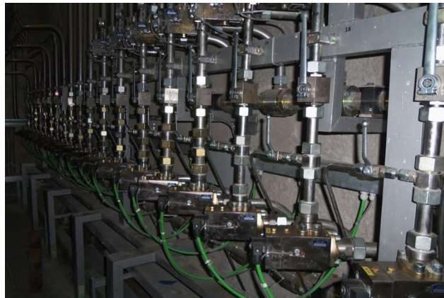
Figure 5.7.3 - Detail of Inox piping and valves of water mist extinguish system @ INFN-LNGS.
